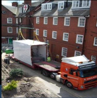
Plant rooms and plant skid
